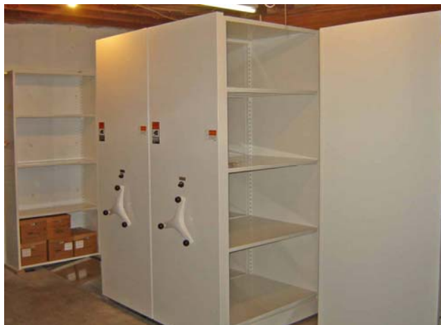
Head-end of PNRA's new Mobile Shelving installation
